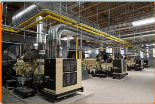
NBC Telemundo Headquarters - Miami, FL (4) 2MW 480v parallel Generators connected to a 6000amp Paralleling Switchgear and (6) Transfer switches to back up (4) Utility services in the building.
