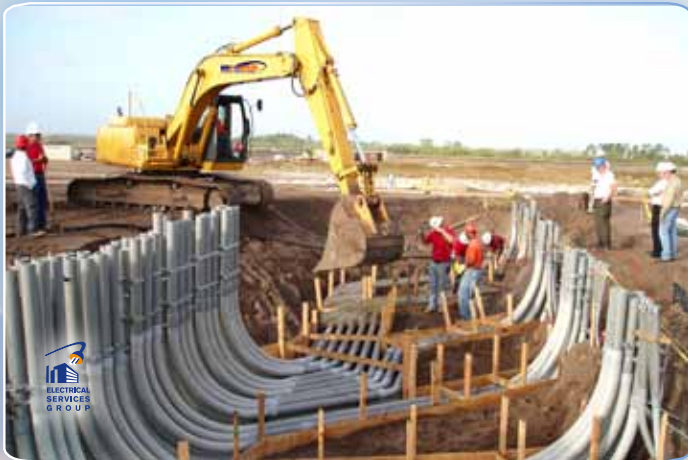
Ave Maria Central Energy Plant Immokalee, Florida
