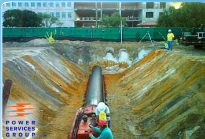
City Center West Palm Beach, FL Duct Bank System Around City Center In Downtown WPB Incorporating & Jack & Bore Across FEC Railway
