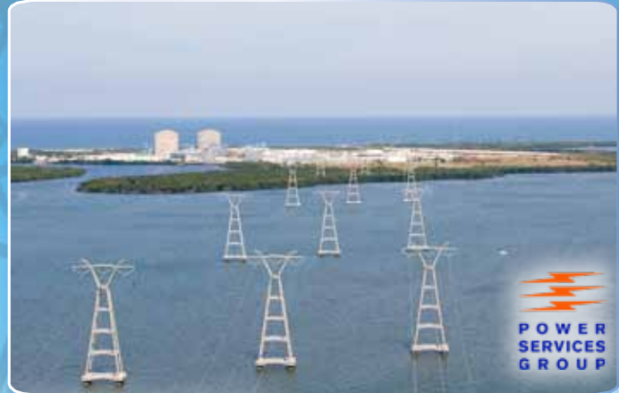
Overhead Power Services St. Lucie, Florida - Replaced hardware and OPGW fiber optic cable on river towers, installed spacers on bundled conductor, replaced guys and anchors.
