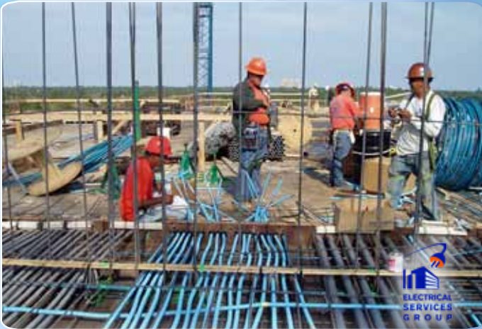
Plaza San Remo Office Building and Parking Garage Coral Gables, FL Complete Electrical Services
