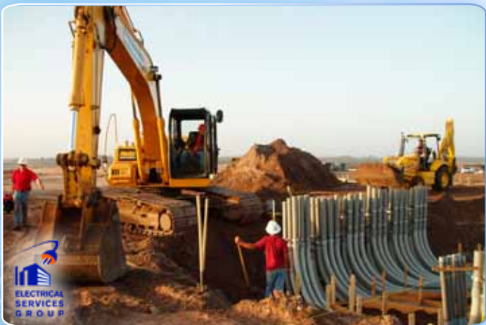
Ave Maria Central Energy Plant Immokalee, Florida
