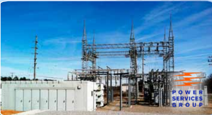
Rock Springs 138/69kV Substation Danville, VA
